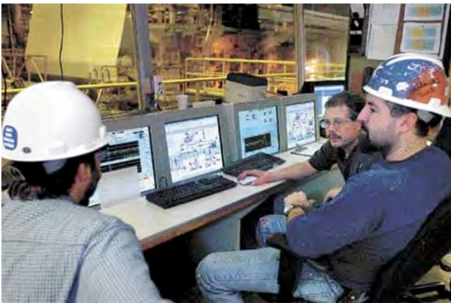
Figure 6. Field diagnostics enables plant personnel to potentially save or extend the life of valuable assets.
