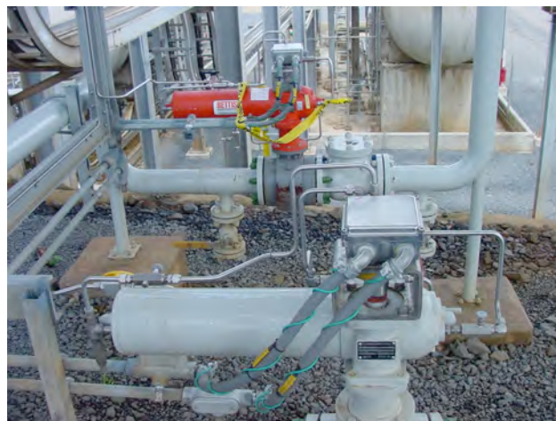
Figure 3. Field device diagnostics help processing facilities practice more preventive and less reactive maintenance.
