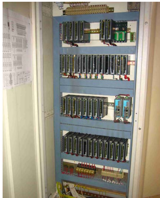
Fig.2: HSE Foundation Fieldbus controller's cabinet
